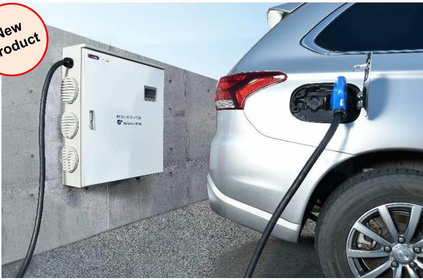
Intermediate capacity quick chargers Example of charging
