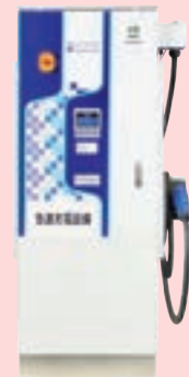
Quick charger connected to an LP gas generator
