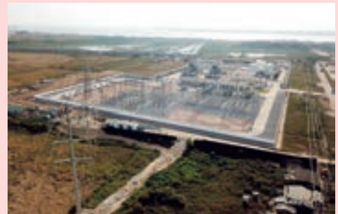
Myanmar Thilawa electrical substation
