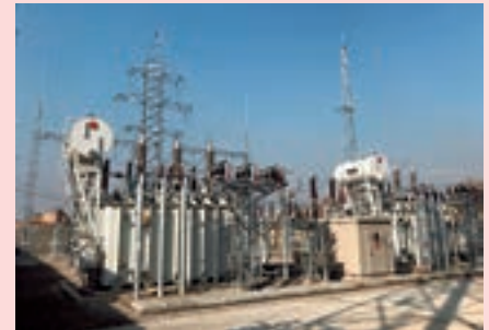
The completed substation in the Republic of Tajikistan
