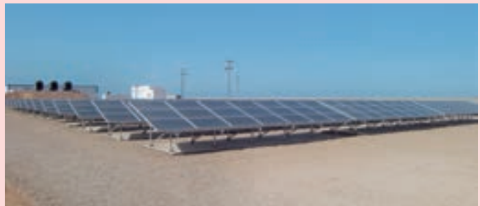
Solar power generation equipment installed overseas
