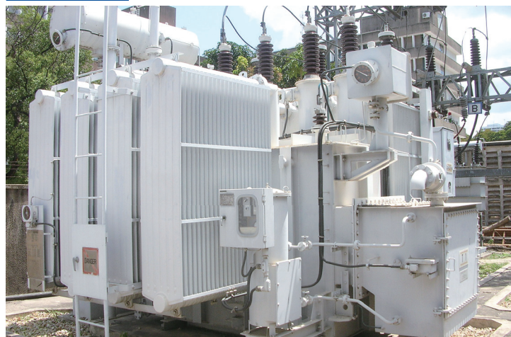
Tanzania (33/11kV 15MVA)
