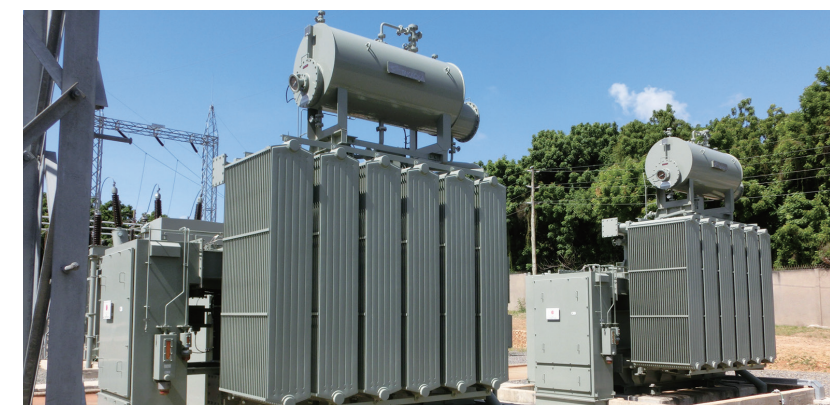
Tanzania (132/33kV 45MVA)
