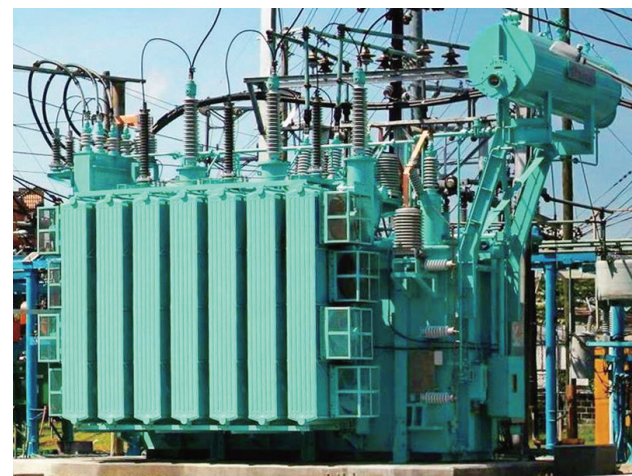
The Philippines (110/34.5/13.8kV 83.33MVA)
