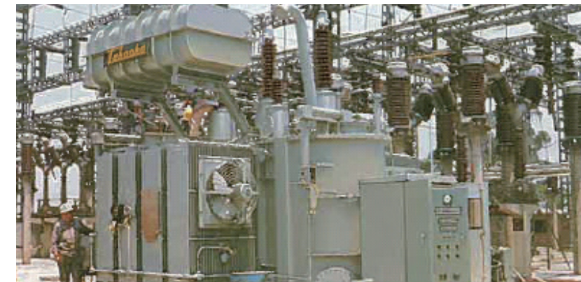
Mexico (85/23kV 30MVA)
