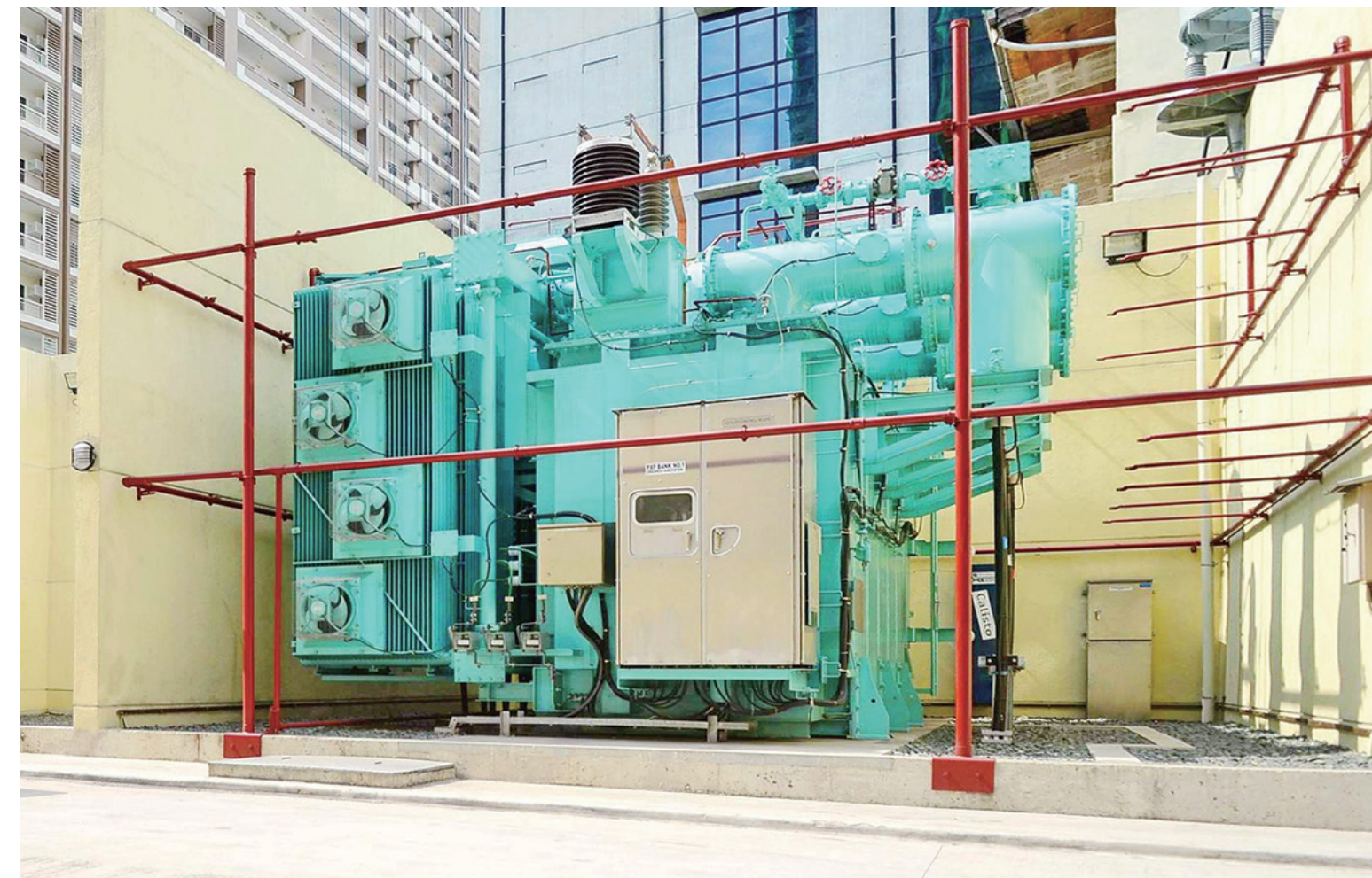
The Philippines (110/34.5/13.8kV 83.33MVA)
