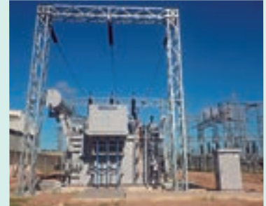
The completed electrical substation in Tanzania
