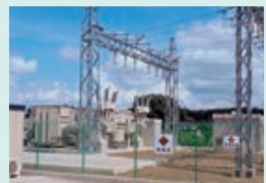
Smart electrical substation
