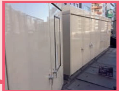
Eco-friendly electrical substation
