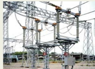
Horizontal center break disconnecter (THB7/8)
